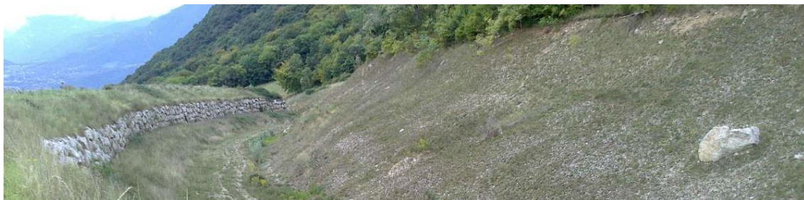
Figure 6. Merlon pare-blocs, (Cerema 2020).
