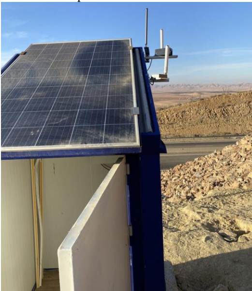
Photo 2. Protective shelters for the installation of management and data acquisition modules
